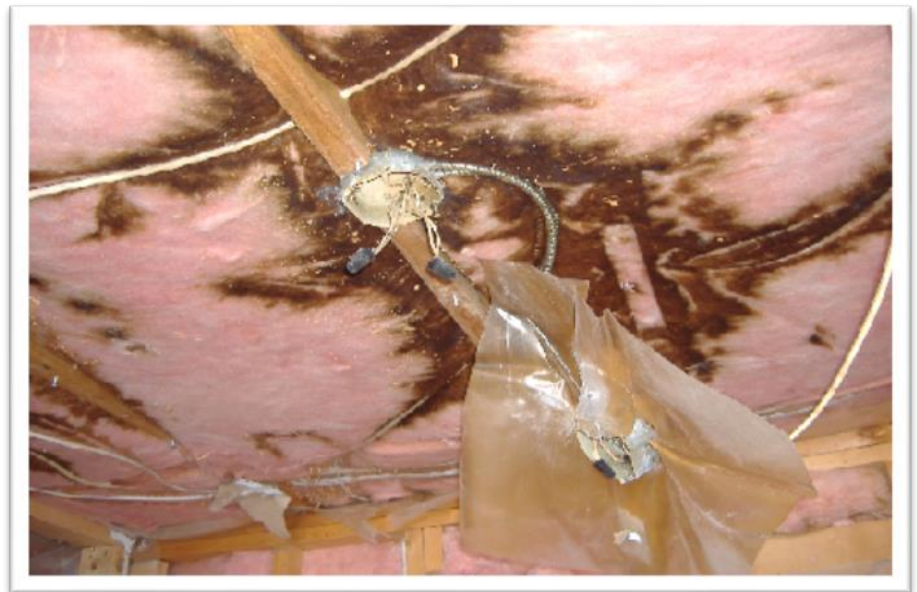
Thirdhand smoke damage to the ceiling of a unit following a decade of chain smoking. Photo courtesy of Haliburton Community Housing Corporation.
